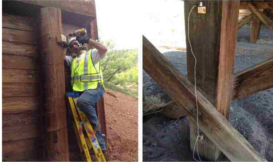
Figure 3-1: Mounting the Wooden Blocks and Attaching the Accelerometers
