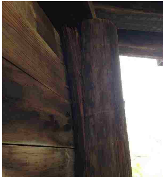
Figure 5-50: Longitudinal Crack Along Pile 14
